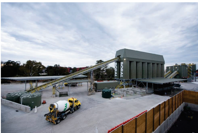
Boral Australia, new West Melbourne Concrete Plant, Vic
