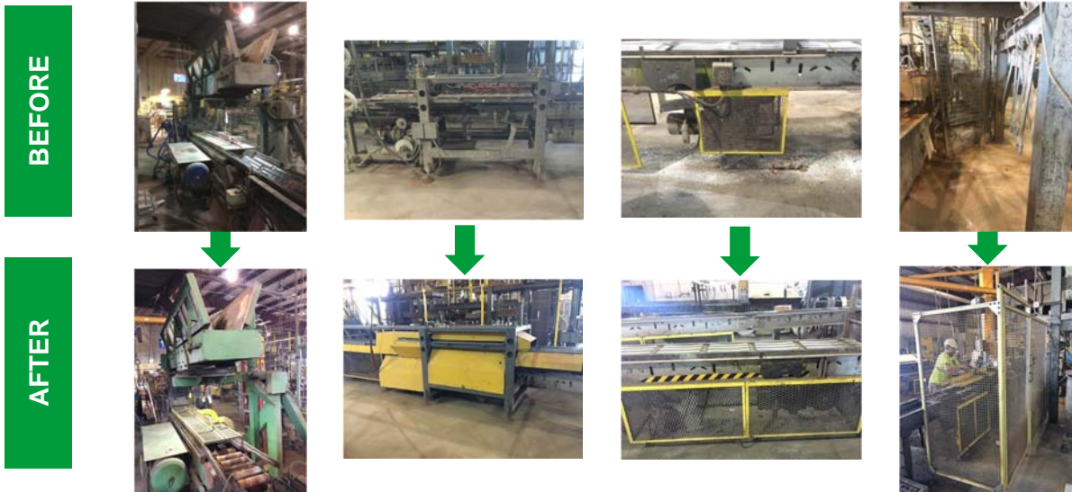
Process flow, access, safety and guarding improvements
