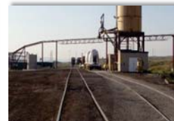
Rail loading system
